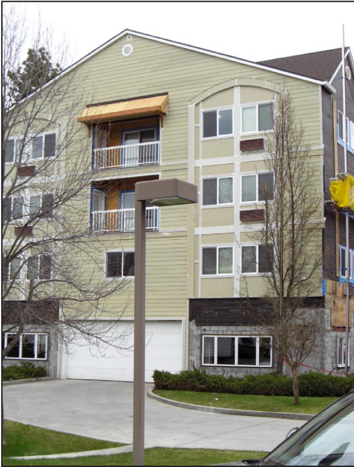
Construction crews are working on the main building's exterior changes. Installation of the cementitious siding has begun. Later exterior changes will include brick accents and a new color scheme.
